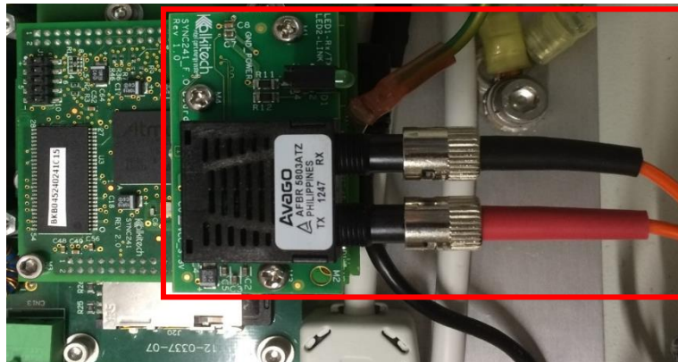
Figure 5-32: Fibre optic module
